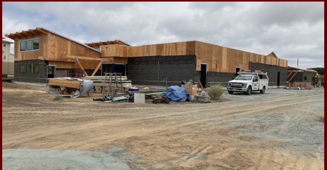
CASTROVILLE Education Center—Work commenced to the application of stucco paper for the exterior finish application June 30, 2021
