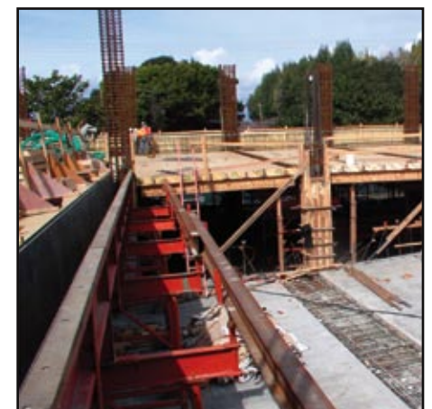
Construction and improvements throughout the campus will bring Hartnell into the 21st century.
